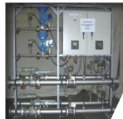
Water / Gas manifold
