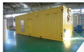
▲ ESS (Energy Storage System)
